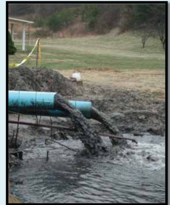
Photo: Oct. 2000 Cleanup of Coal Sludge Spill
